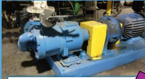
Stage 1 CM Pumps, Compressors
