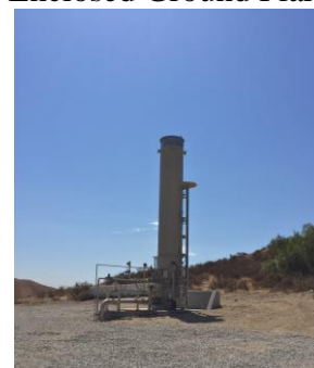
Enclosed Ground Flare
