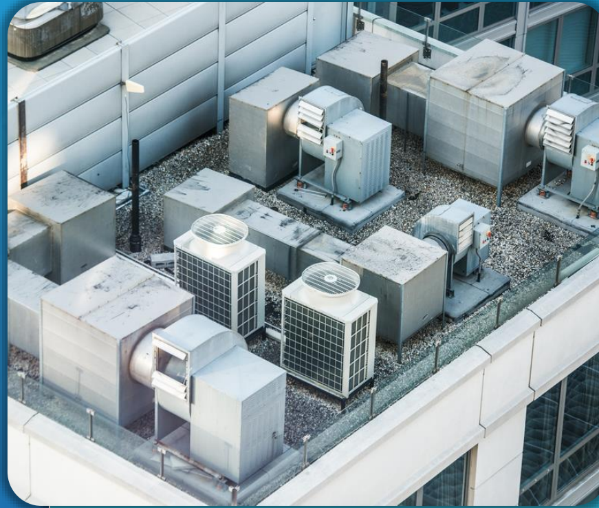
Commercial Combustion Water/Space/Heating/Cooking/ Others
