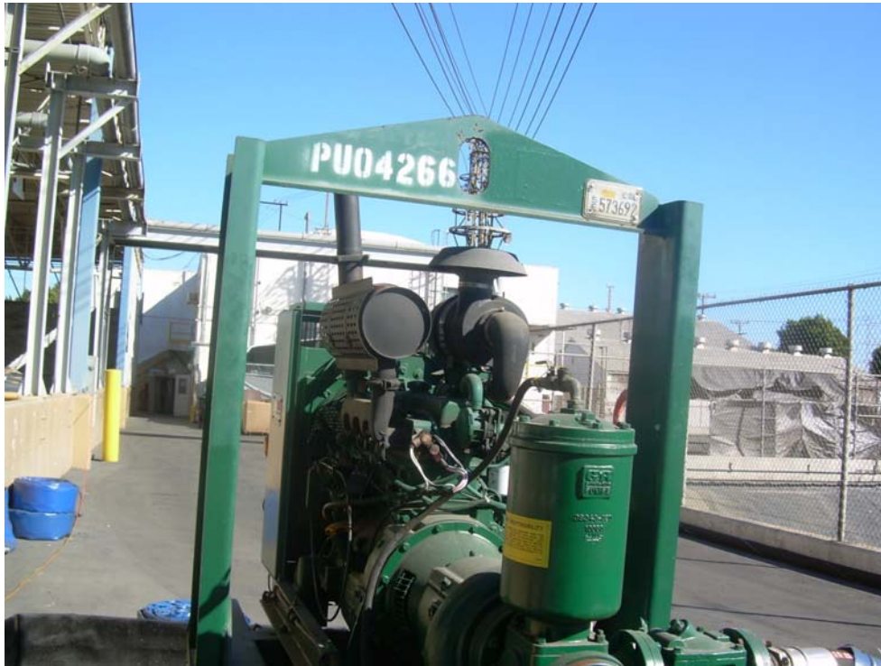
Existing Pump for Temporary Storm Water Management System Figure 3-5
