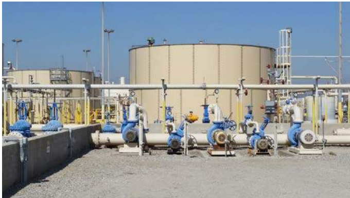
Figure 1-7. Storage Tanks at the 700 Block Main Facility. Similar to those that will be a part of Proposed 400 Block Reinjection Facility. For full size, see Figures section at the end of the Chapter 1.
