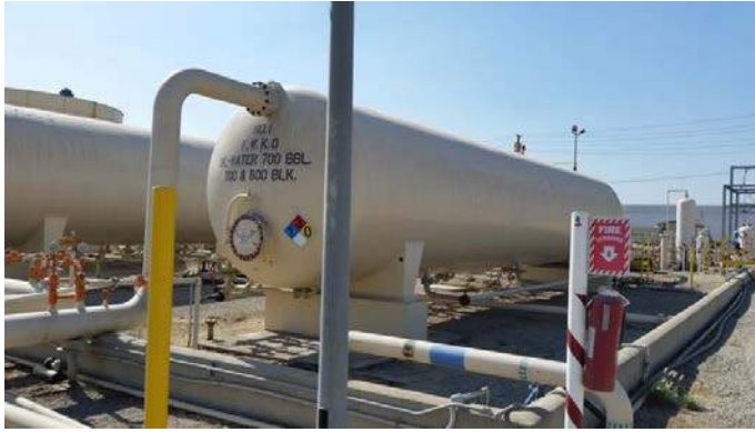
Figure 1-6. Free Water Knock Out Vessel at the 700 Block Main Facility. Two comparable Free Water Knock Out Vessels will be included at proposed 400 Block Reinjection Facility. For full size, see Figures section at the end of the Chapter 1.
