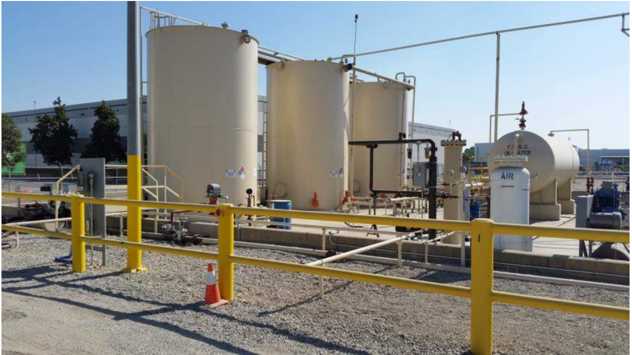
Figure 1-8: Existing Truck Loading connection in the foreground of the Baker Humble tank, located at the 700 Block. The proposed new connection would be added immediately adjacent to existing connection.
