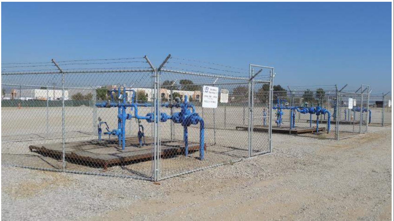
Figure 1-15: Typical water injection well located at 700 Block.
