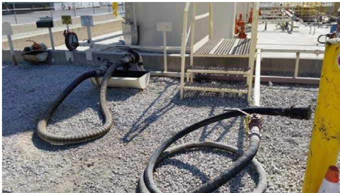
Figure 1-12. Existing Truck Loading Connection/Hoses at 700 Block.
