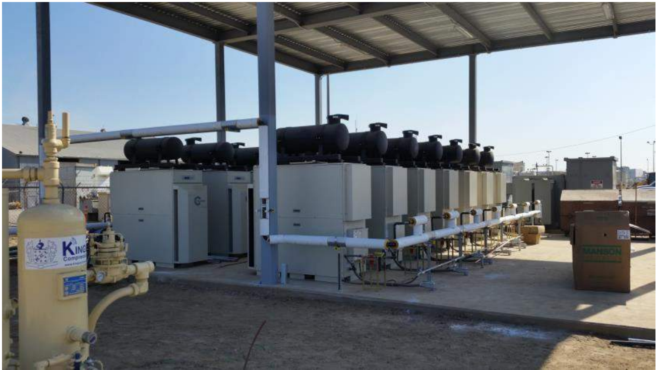
Figure 1-16: Breitburn's microturbines, which have been installed but are not yet operational. Noise dampers are visible on the top of each turbine.
