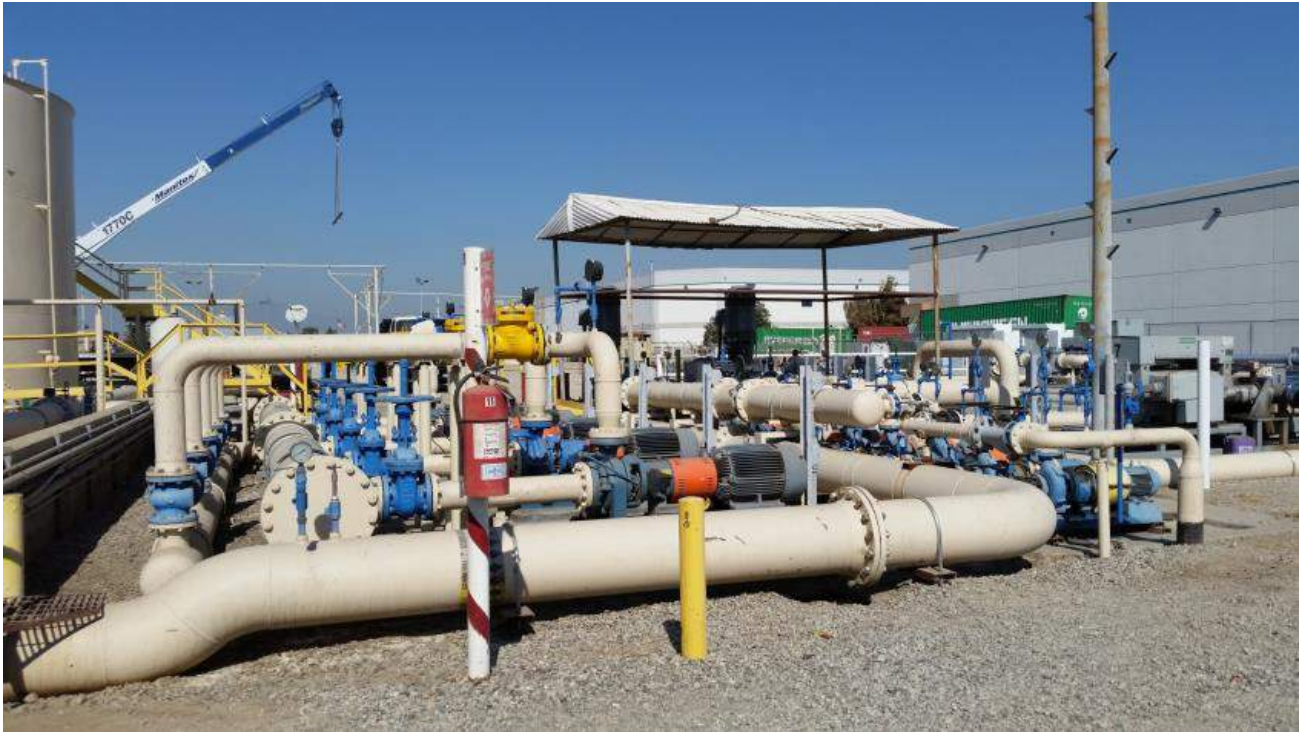
Figure 1-11: 700 Block Main Facility pump and ancillary equipment area.
