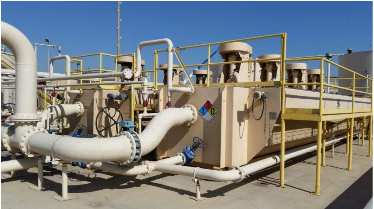
Figure 1-9: 700 Block – WEMCO separator at the 700 Block Main Facility, similar to that which will be installed at the proposed 400 Block ReInjection Facility.
