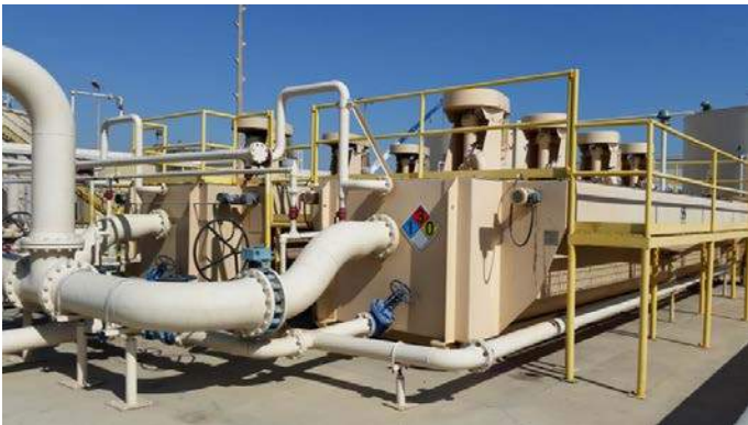
Figure 1-9. WEMCO Separator at the 700 Block Main Facility.
