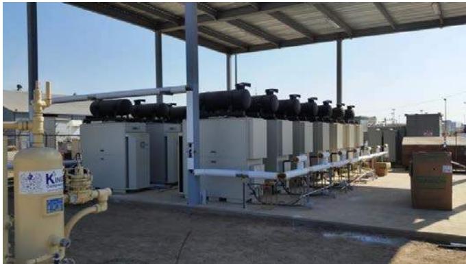
Figure 1-16. Breitbart's Microturbines. These have been installed but are not yet operational. Noise dampers are visible on the top of each turbine. For full size, see Figures section at the end of the Chapter 1.
