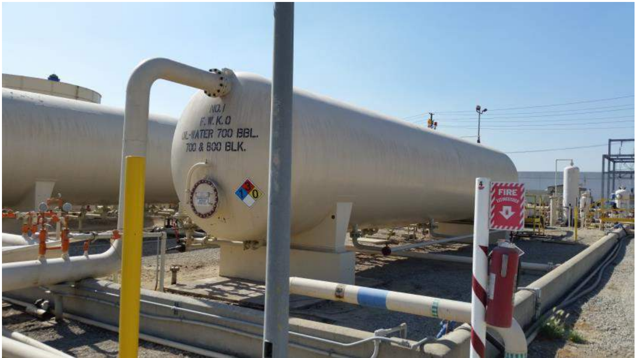
Figure 1-6: Free Water Knock Out Vessel that is part of the 700 Block Main Facility. Two comparable Free Water Knock Out Vessels will be included at proposed 400 Block ReInjection Facility.
