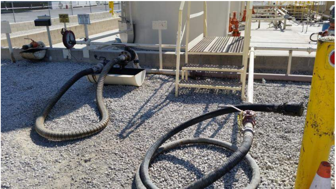
Figure 1-12: Existing Truck Loading Connection / Hoses at 700 Block. The proposed new connection would add additional hoses and vapor recovery lines such that trucks could be loaded simultaneously.
