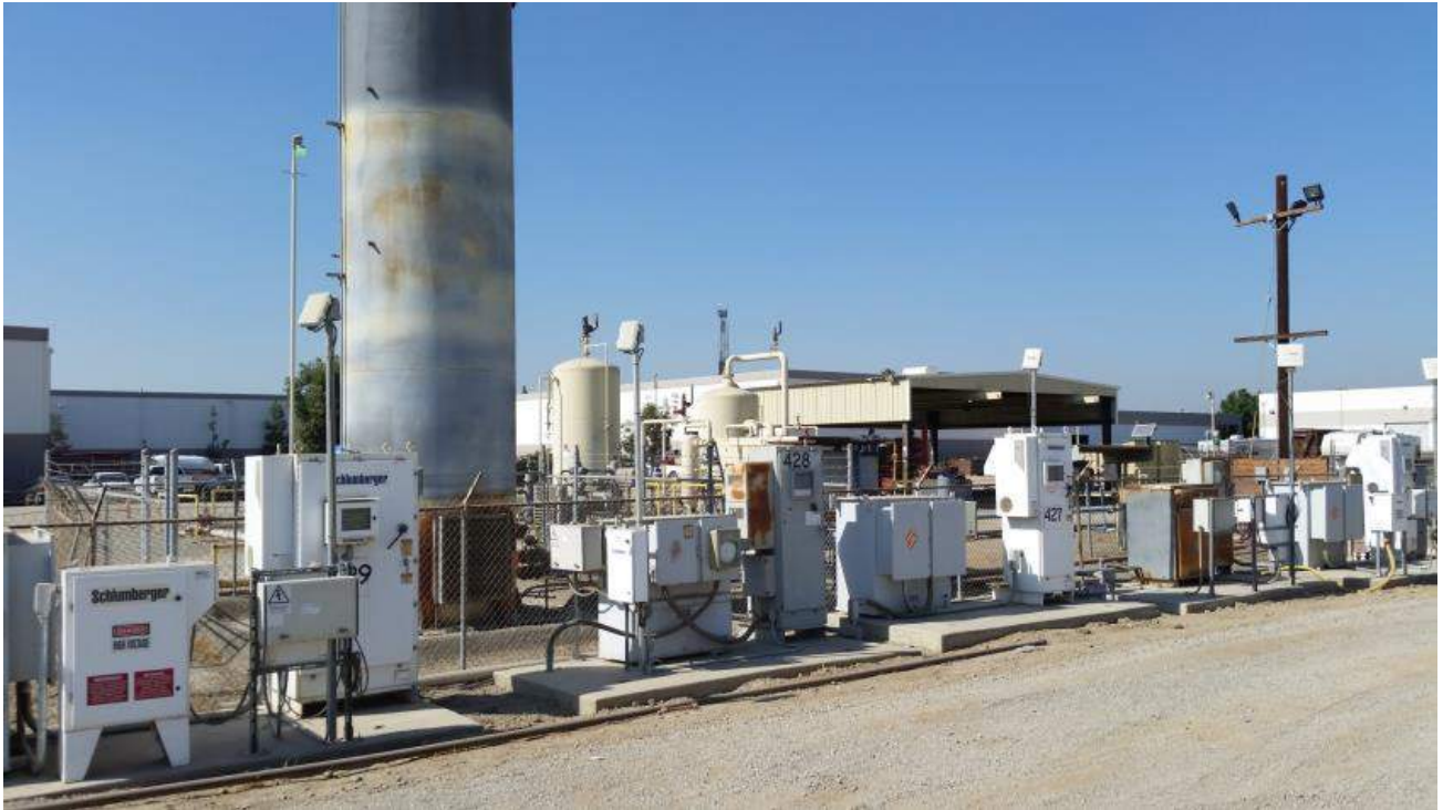
Figure 1-13: Existing Flare, located at the 400 Block, will be replaced with new, low emitting flares in the same location.
