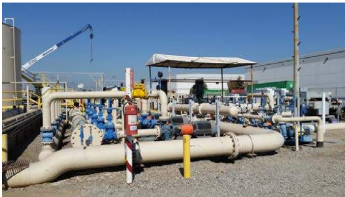
Figure 1-11. 700 Block Main Facility Pump and Ancillary Equipment Area.
