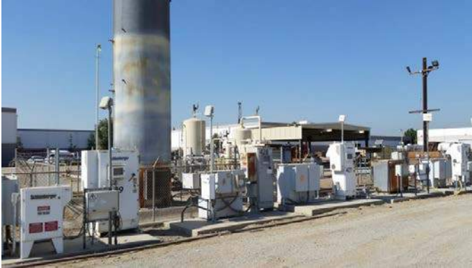
Figure 1-13. Existing Flare Located at the 400 Block. This will be replaced with new, low emitting flares in the same location. For full size, see Figures section at the end of the Chapter 1.
