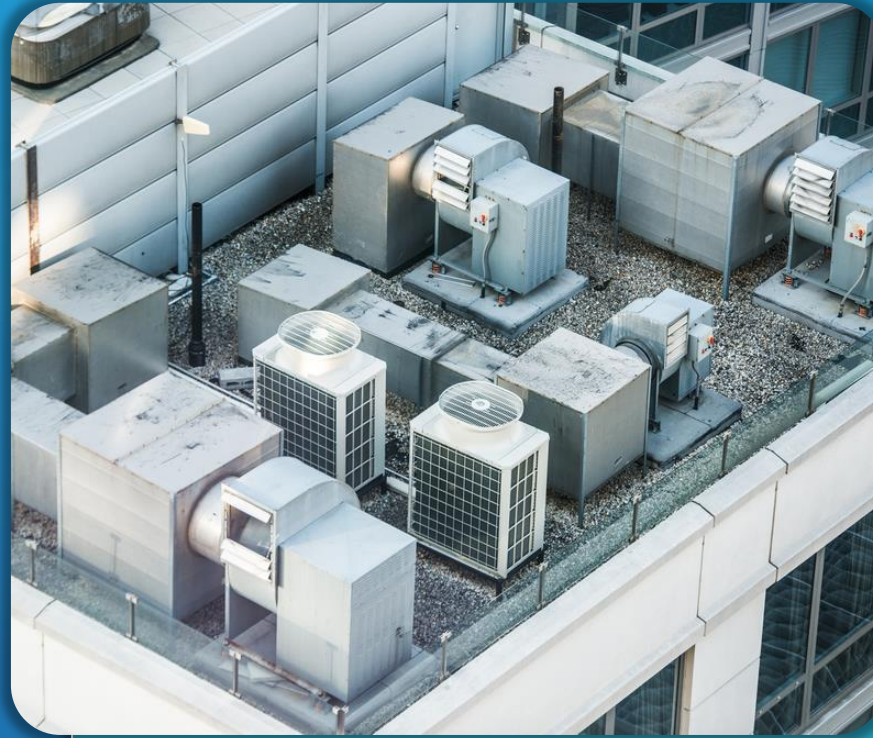
Commercial Combustion Water/Space Heating/ Cooking/Others
