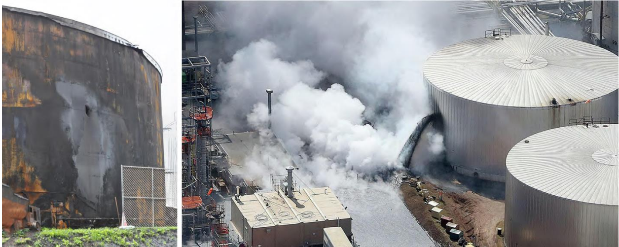
Figure 5 — Enormous hole several feet in diameter in an asphalt storage tank resulting from the April 26, 2018 Husky Superior Refinery Explosion in Superior, Wisconsin.
