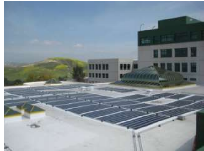
BIPV by Solar Integrated
