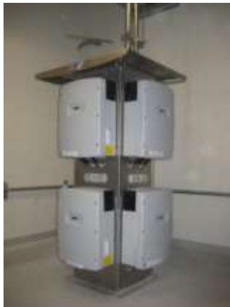
ST-42 Inverter Tree Used by Both Systems
